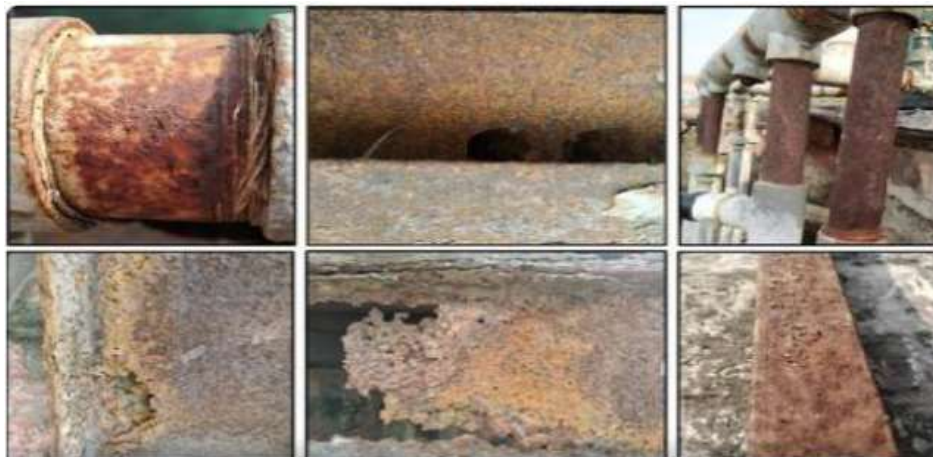
Figure IV-1 Effects of corrosion on different metallic structures
