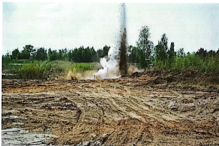
Figure II.13. View of an explosive compaction site at the moment of detonation, Gdansk – Poland (Ménard Polska)
