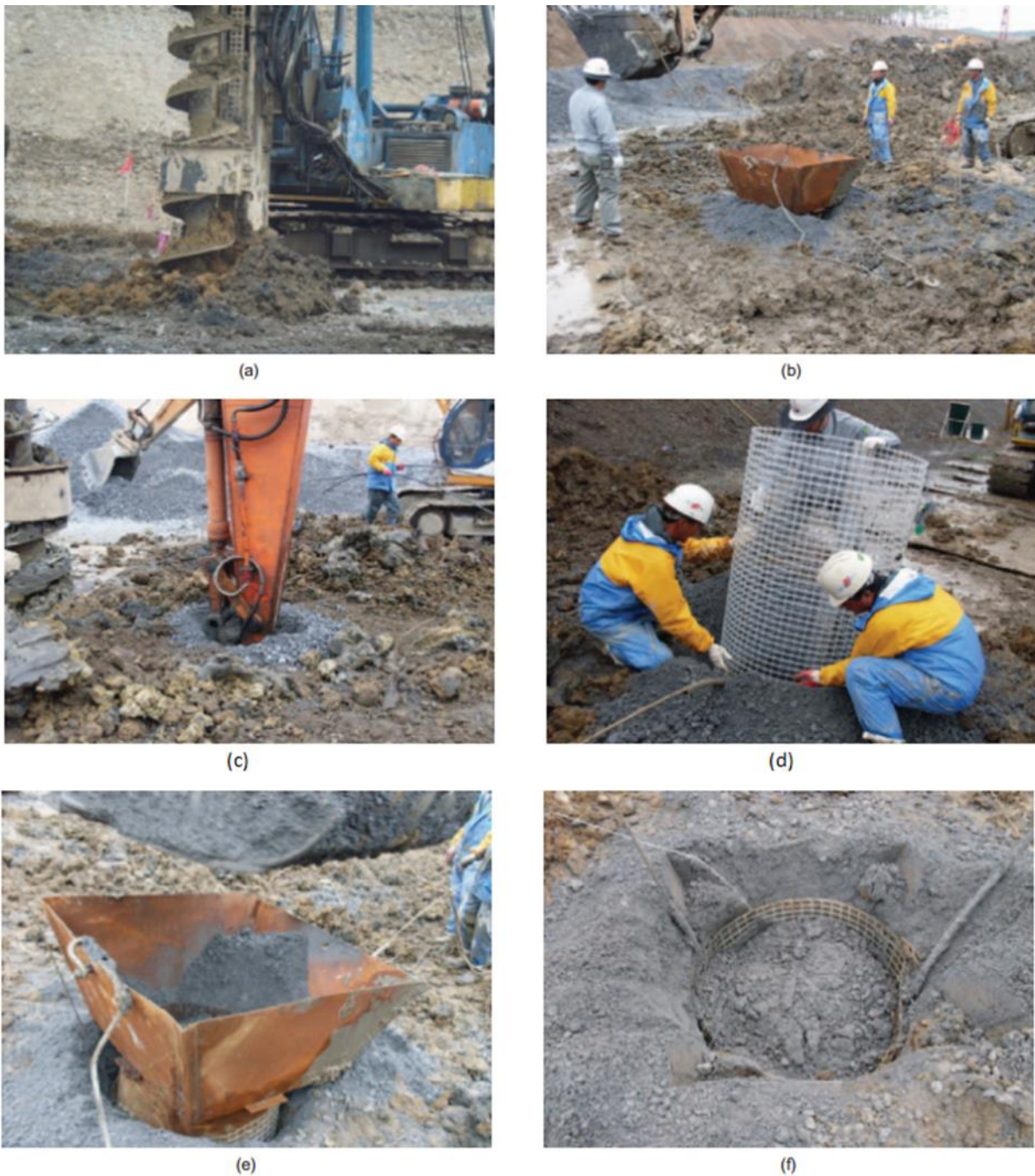
Figure 2-30. GESC installation: (a) auger is used to remove soil; (b) insertion of aggregate by funnel; (c) compaction of aggregate; (d) geogrid sleeve is placed; (e) insertion of aggregate into geogrid sleeve; (f) GESC installation is completed (Yoo and Lee, 2012).
